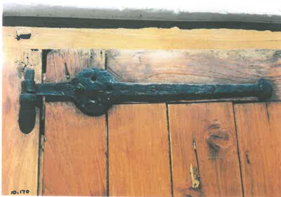
50. The exposed woodwork has suffered much at the rear. These casements and shutters should be oiled, sealed and painted. The pintle is recent (>1950) and the straphinge old (18 th century).
