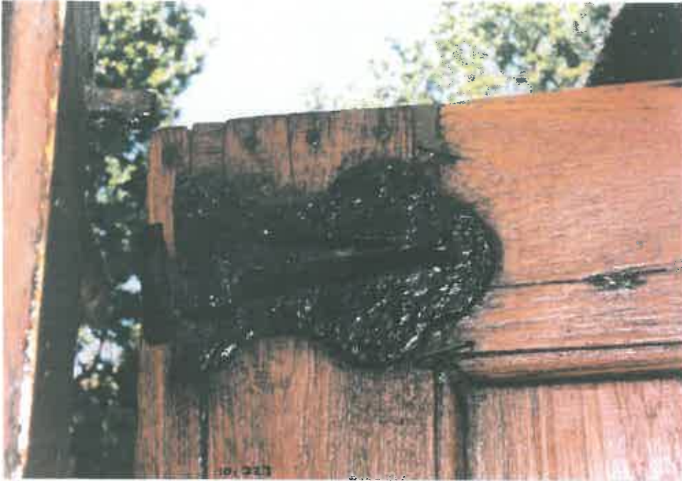
52. A shutter spring-latch, but in poor condition.
