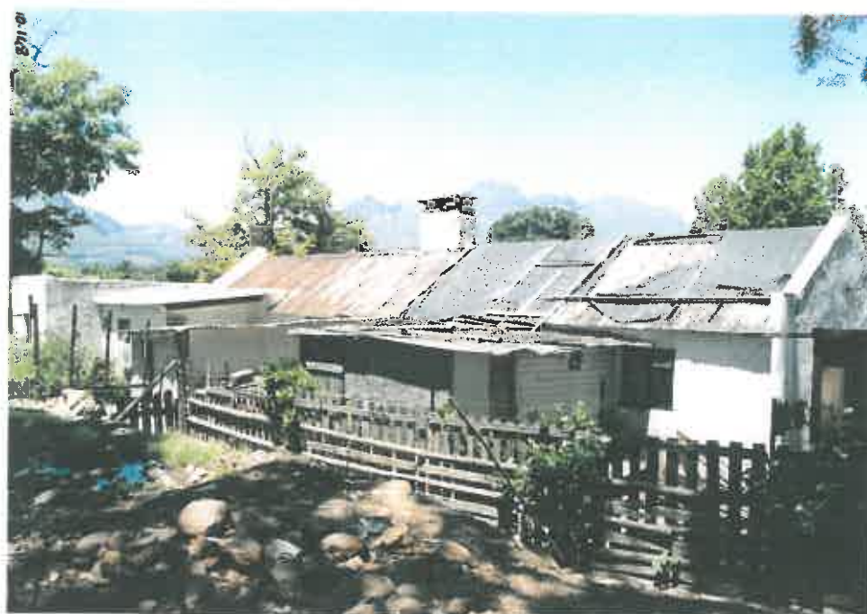
147. The second binary cottage, with a roof that greatly leaks. Author judges them to be of the second half of the 19 th century, but they need a thorough inspection.
