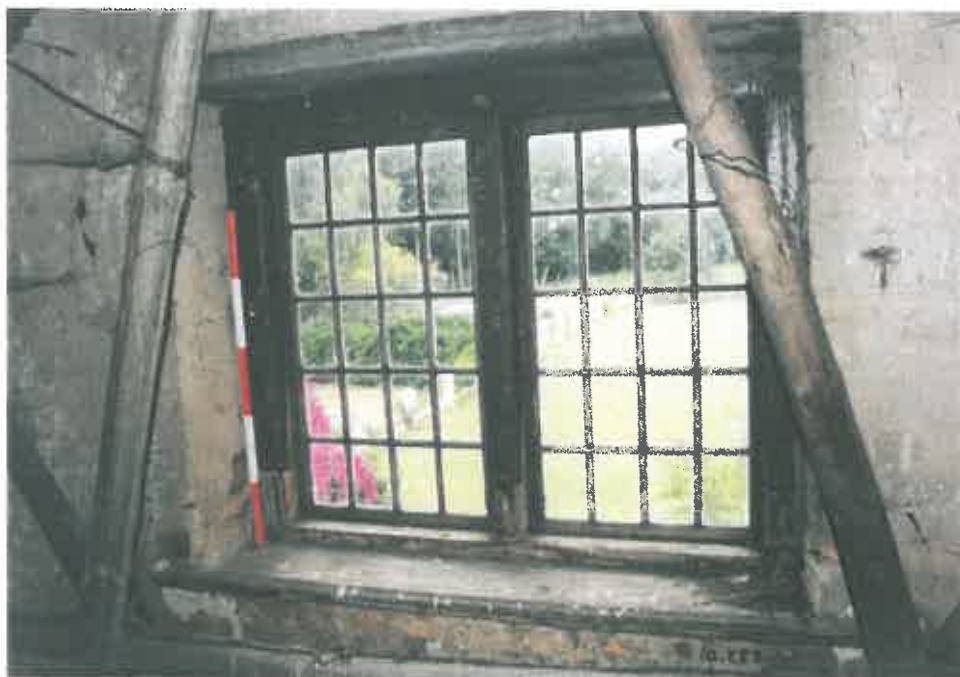
73. The dormer casement in the rear gable is exactly similar to the one in front. Signs of charring was visible.
